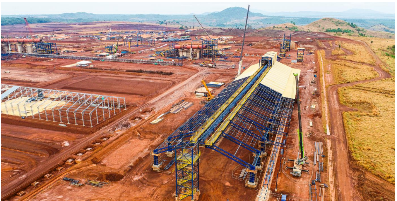
All the structural steelwork is in place on the ore homogenisation building, with the cladding of the roof underway.
