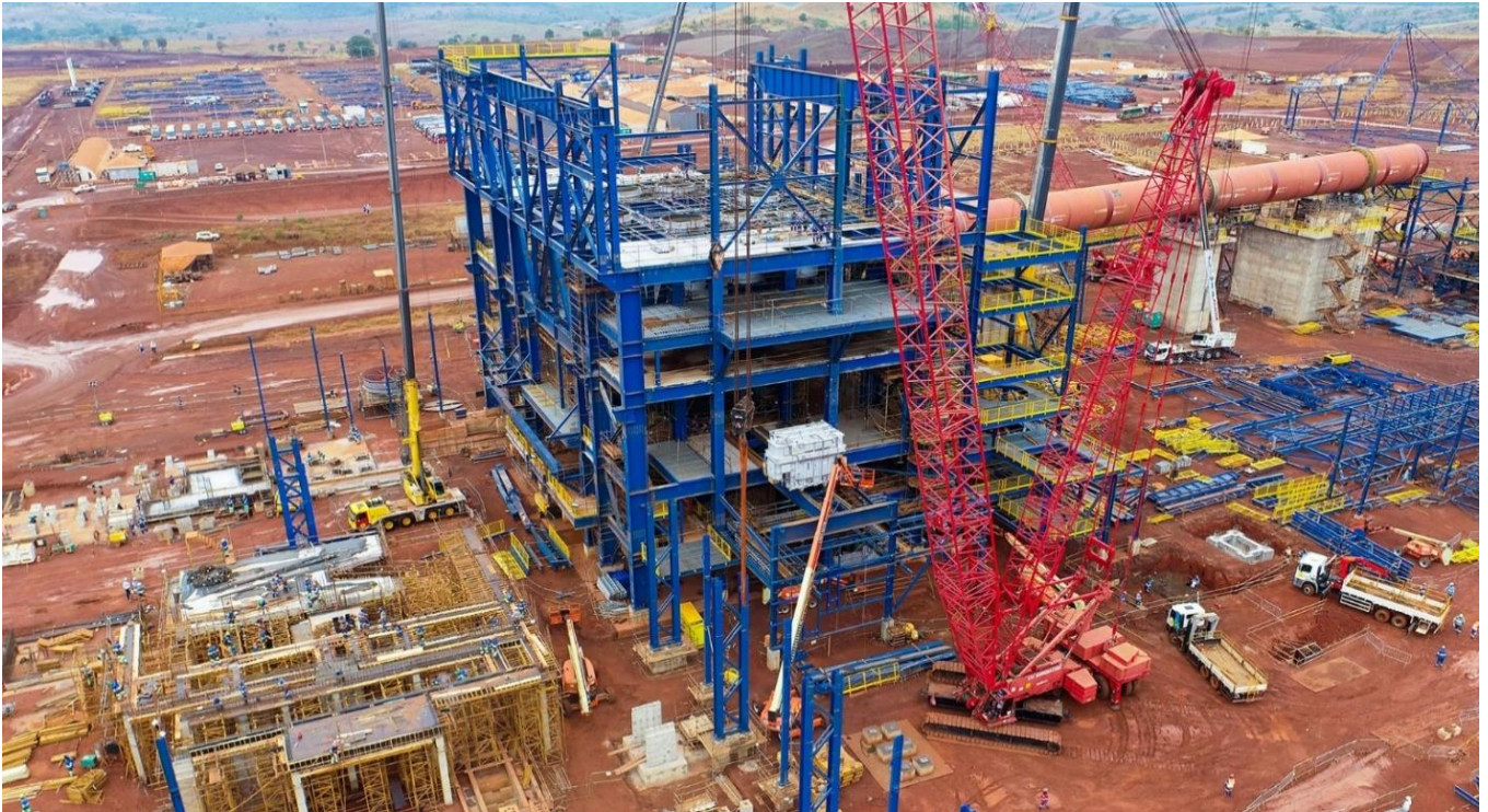
The Electric Arc Furnace building in the centre with the electrical transformer being positioned on the second level, to the left of the image is the refinery building.
