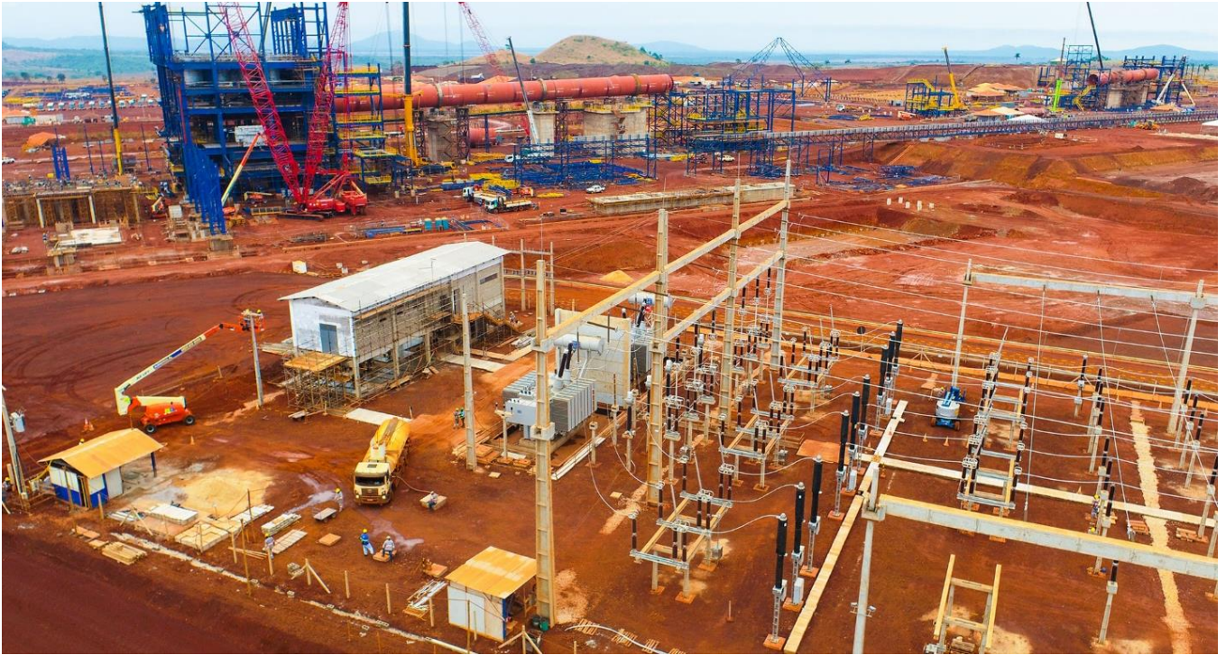
The Araguaia sub-station with both of the main 230kV/34.5kV transformers installed.
