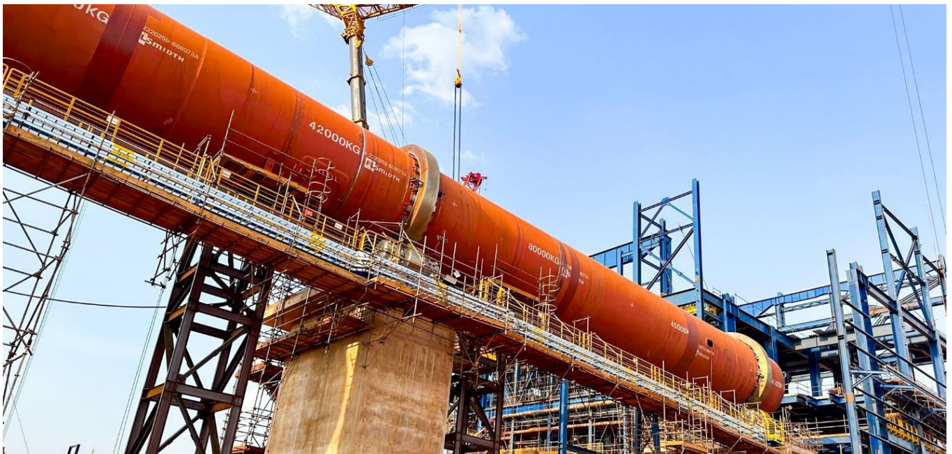
The Rotary Kiln installed on the support piers with main roller bearing guide rings visible.
