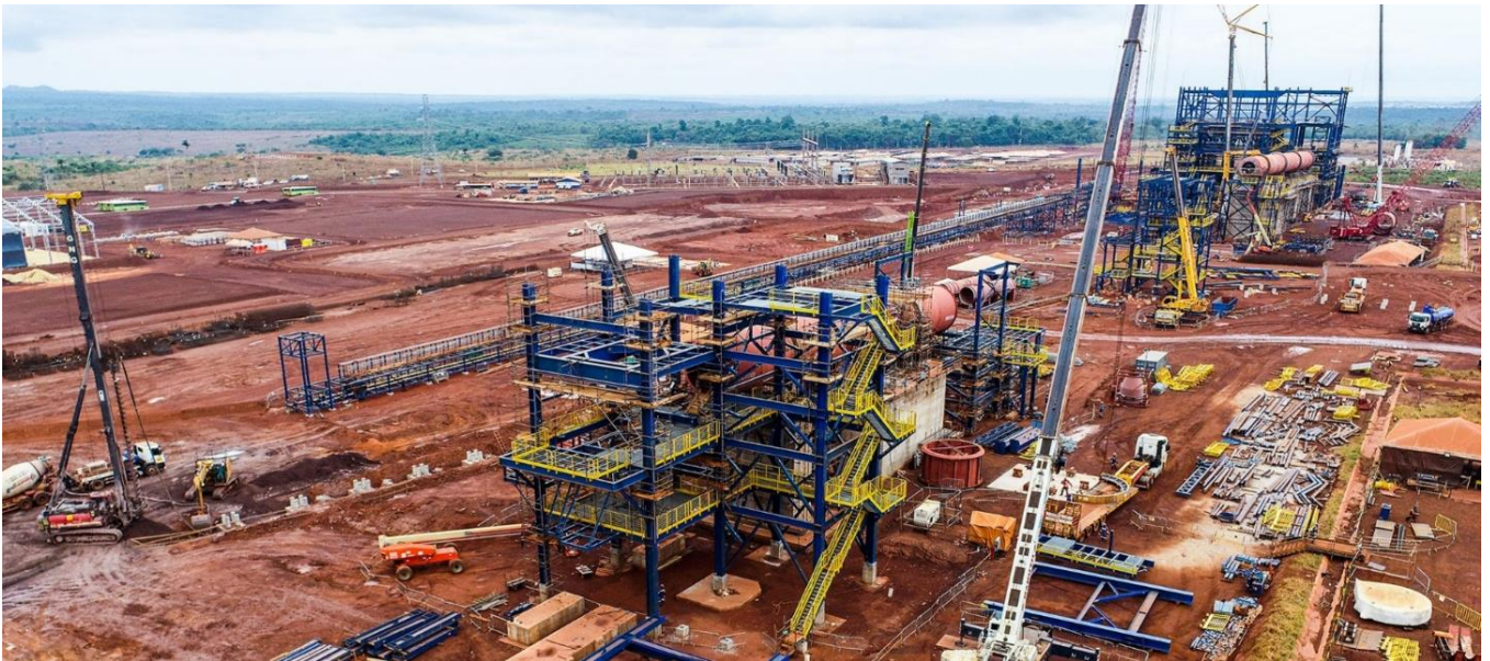
The Rotary Dryer (foreground) is scheduled for commissioning by year end.
