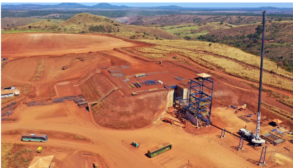
Figure 2 – The ROM pad, ROM bin and primary crusher
