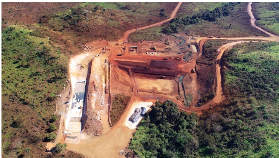
Figure 8 – Water storage reservoir
