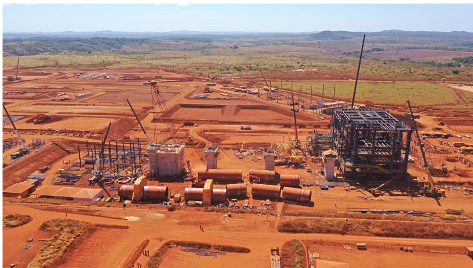
Figure 4 – Rotary kiln piers, the individual kiln pieces, the steel erection of the electrostatic precipitator and the electric arc furnace
