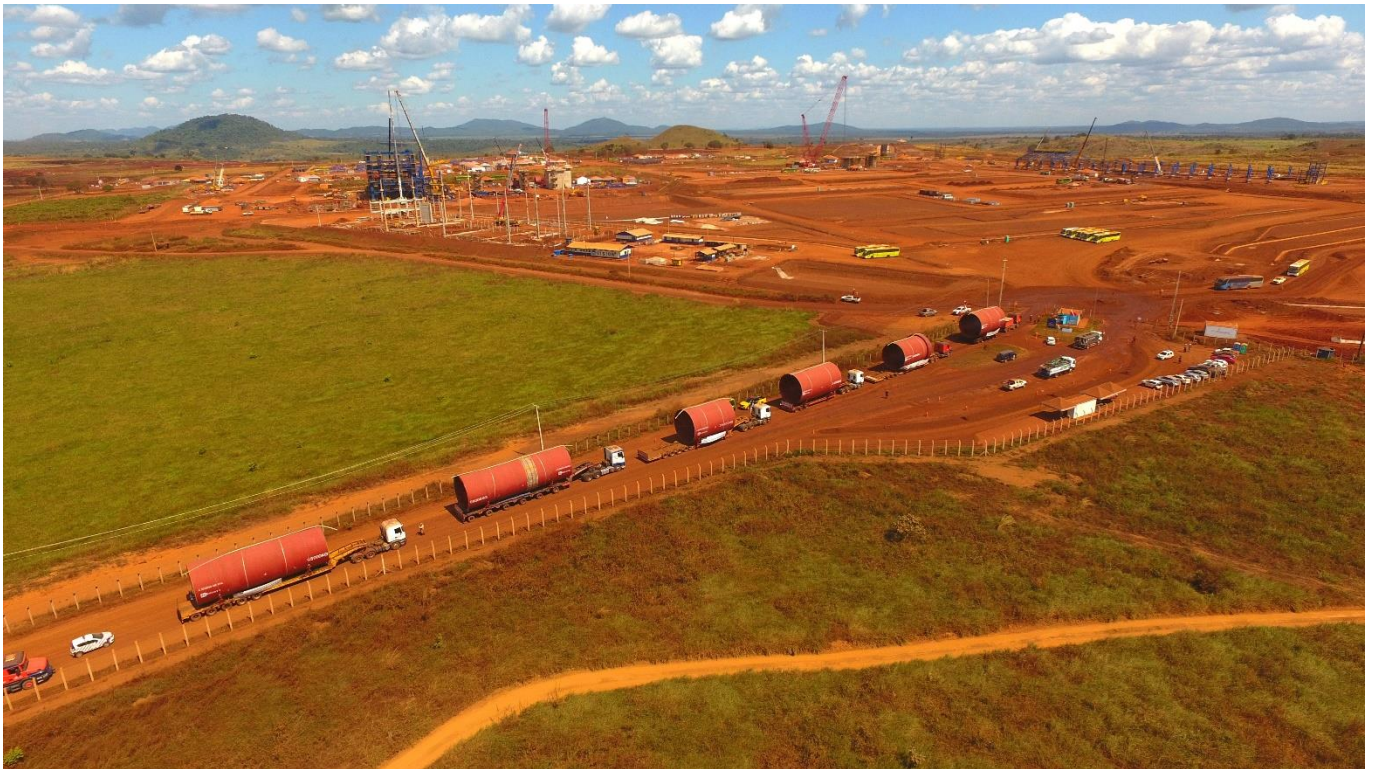
Figure 2: The rotary kiln arriving at the Araguaia Nickel Project. The individual sections of the kiln will be welded together over the course of the next month before being lifted into place and aligned on the kiln piers.
