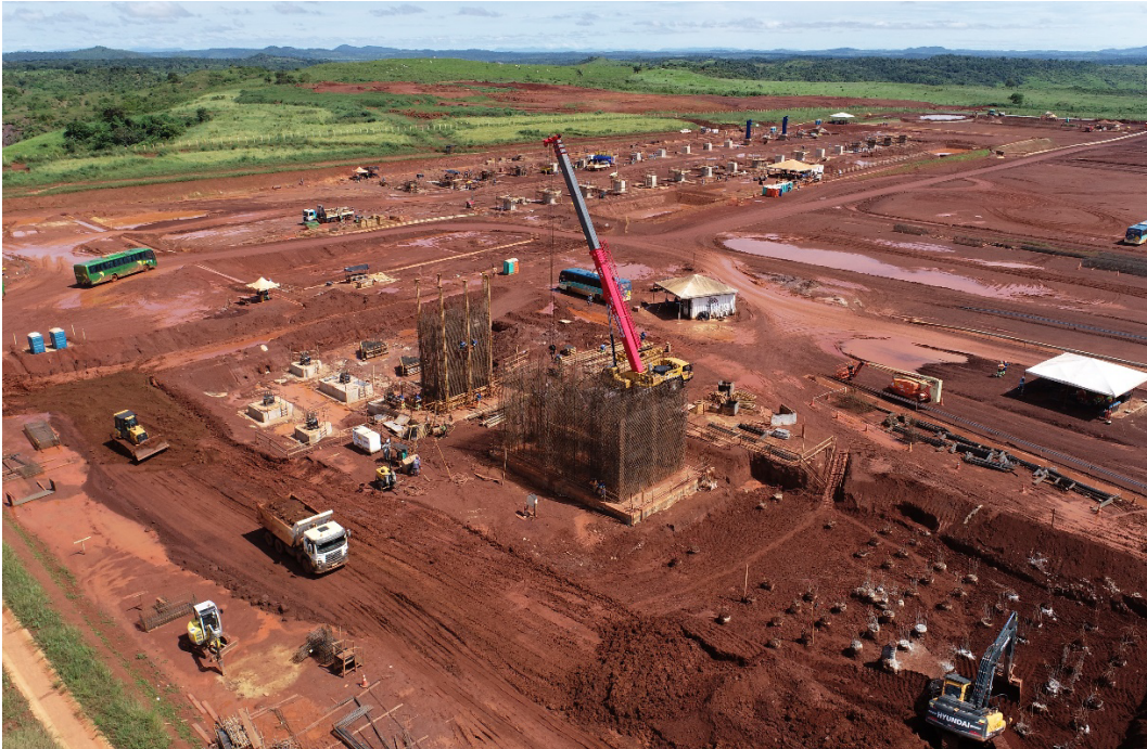
Figure 3: Foundations of the dryer support columns, showing steel form work ready for the application of concrete.
