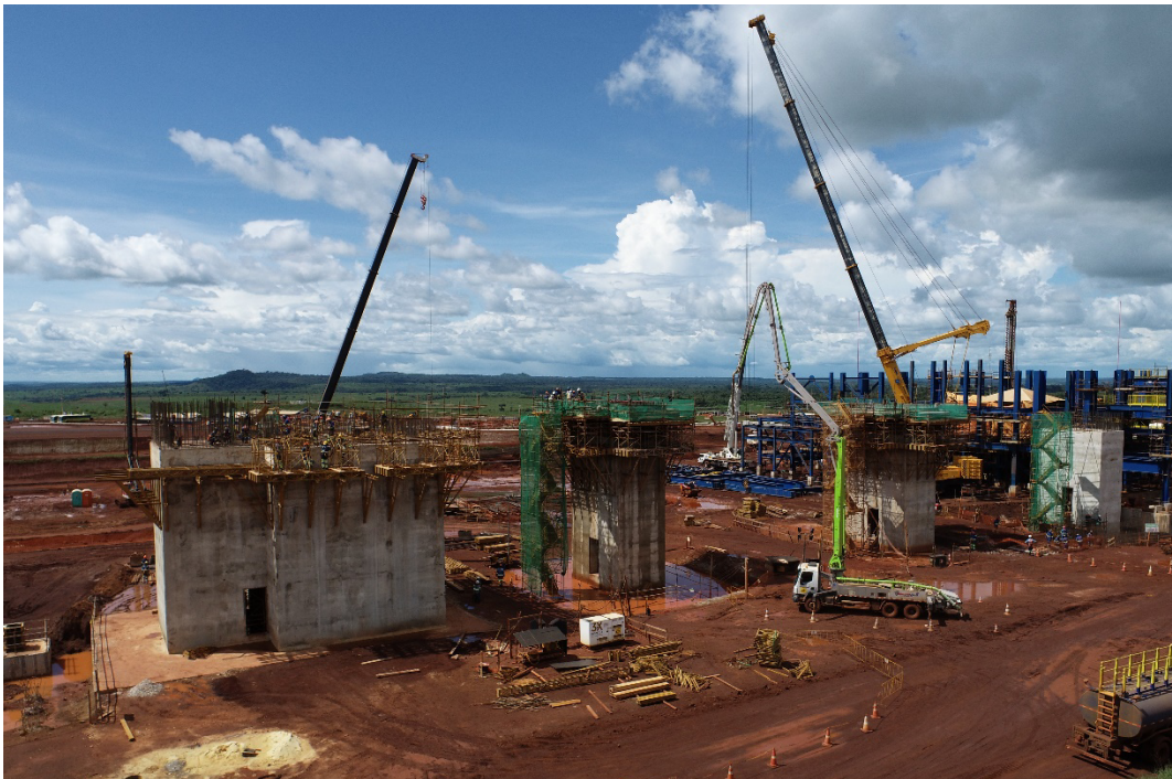
Figure 2: The four 6m high columns to support the Rotary Kiln, showing the slip forms in place to cast the top cap sections.
